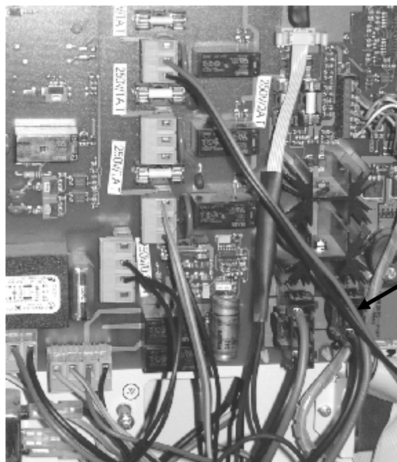
connectors on the power board
